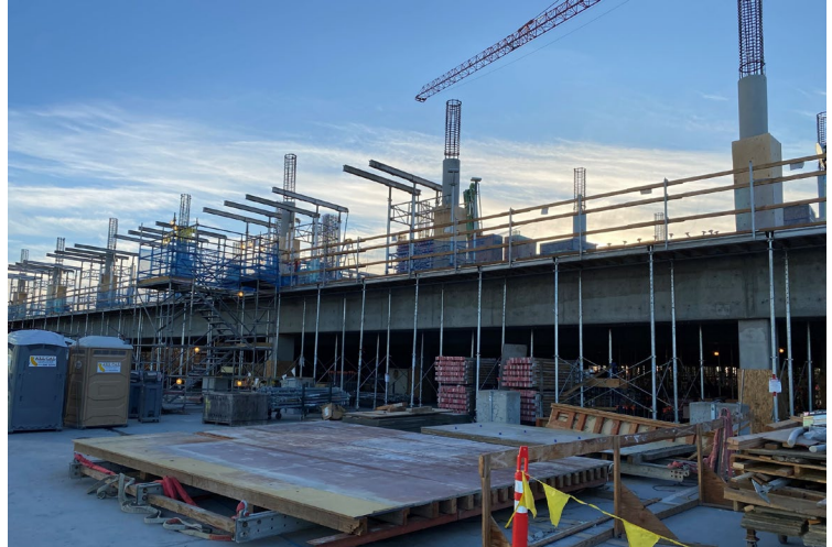
View of the first office level on the 6th floor from Phase I parking level
